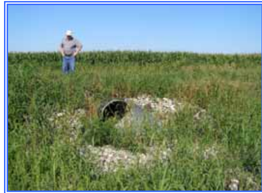
Ted inspecting a new seeding along an open ditch. Note: side inlet pipe that serves as an outlet for a waterway.
