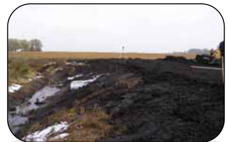
Ditch bank now re-shaped and new pipes installed. Large pipe is for surface water and smaller pipe is for tile water.
