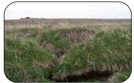
This gully problem existed in the ditch bank prior to the installation of the new Side Inlet Pipe.
