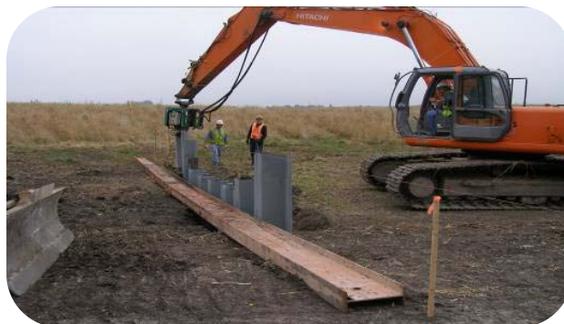
Driving steel sections of a Sheet Pile Structure. Backhoe on right, Steel I beam on ground, string for
