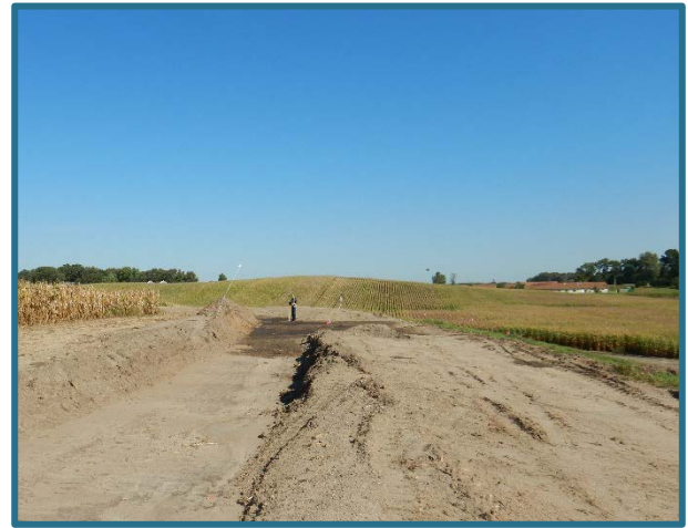
SWCD Technician Jarod Schamaun checking on a structure which was under construction during a large rain event.
