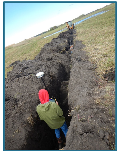
SWCD Technician Jarod Schamaun making sure a wetland restoration is meeting NRCS specs and standards before the contractor closes the trench.
