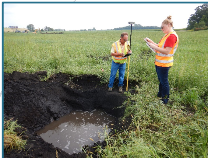
NRCS Civil Engineering Technician (CET) Joseph Christensen and SWCD Technician Lindsey Zeitler making sure a tile break is meeting NRCS specs and standards.
